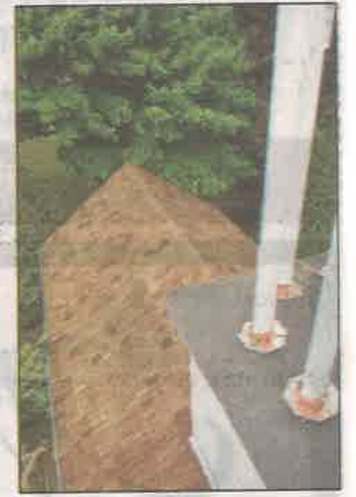
View from the new-old tower. Master craftsman Jeff Haynes of J&R Haynes LLC milled new columns to replace the decaying ones, chiseling them to within an eighth of an inch of the original.
