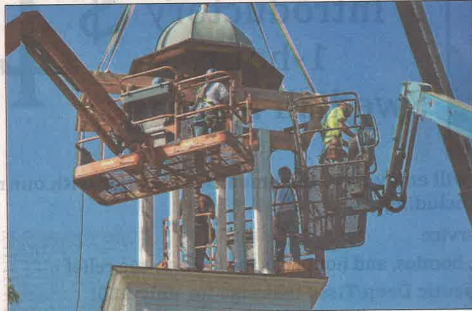
Easy does it — construction crew works to place the bell tower just right.
